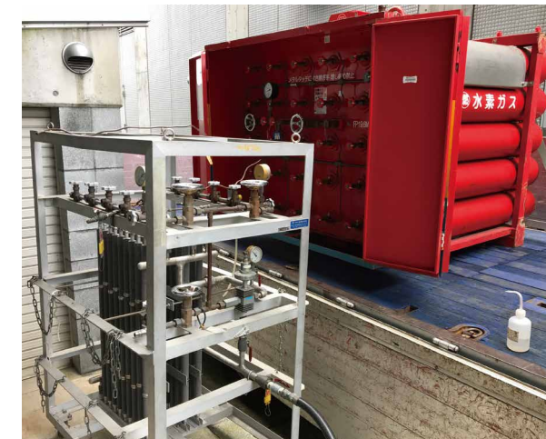
Photo 3-3 Hydrogen cylinder bundle (in rear of the photo)
