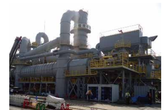
Photo-10 General view of preheating kiln of NTR-Stage VI
