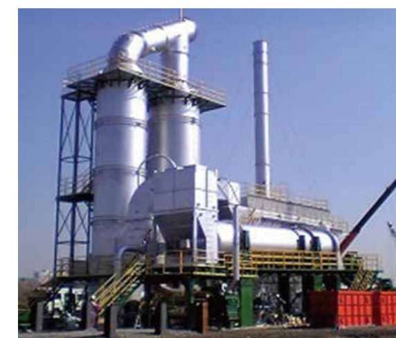
Photo-7 General view of NTR-Stage IV plant
