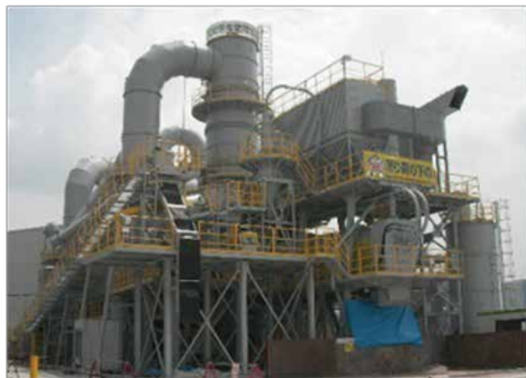
Photo-9 General view of NTR-Stage VI plant
