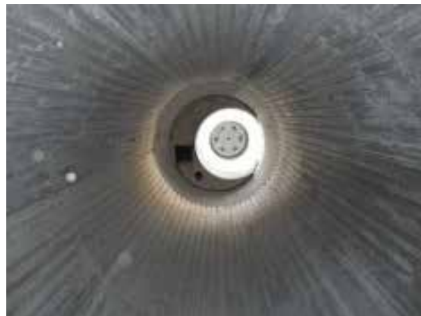
Photo-15 Interior of primary treatment device of NTR-Stage VI
