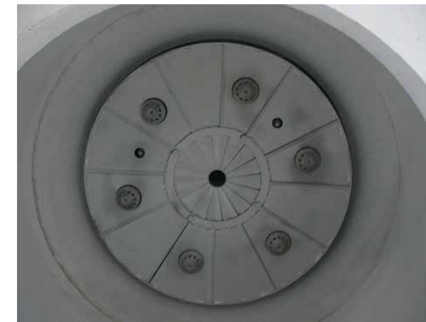
Photo-18 Interior of burner of primary treatment device of NTR-Stage VI
