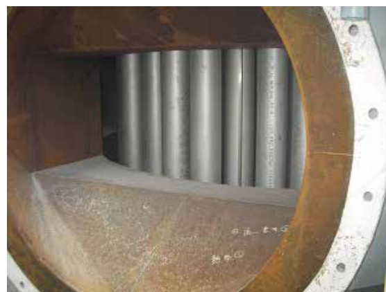
Photo-16 Heat-receiving gas inlet on side of heat exchanger of NTR-Stage VI
