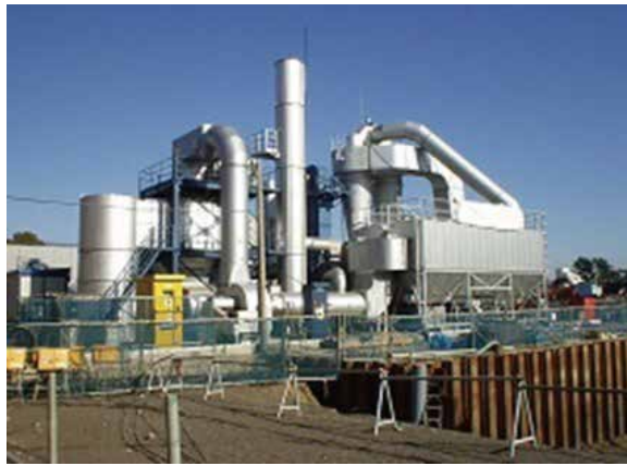
Photo-5 General view of NTR-Stage II plant
