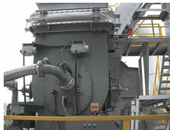
Photo-17 Preheated air burner of primary treatment device of NTR-Stage VI
