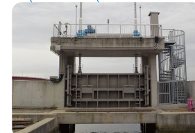
Floodgate (Other Business)
