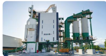
Asphalt plant (AP-Related Business)
