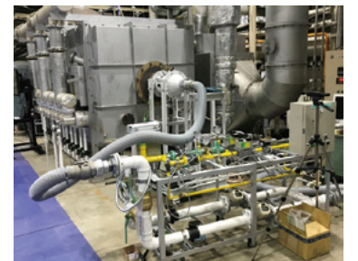
Hydrogen burners (in development)
