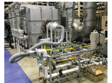
Hydrogen burners (in development)
